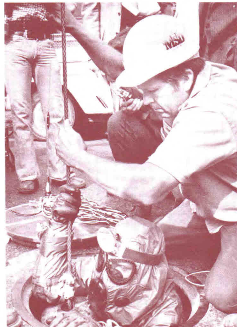
The illegal dumping of a toxic substance into the Louisville sewer system necessitated a time-consuming and costly cleanup.
